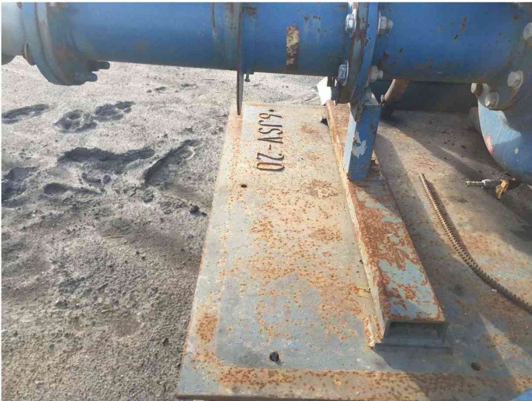
Figure 4 – Photographs of Unit 2 Slurry Pond Pump
